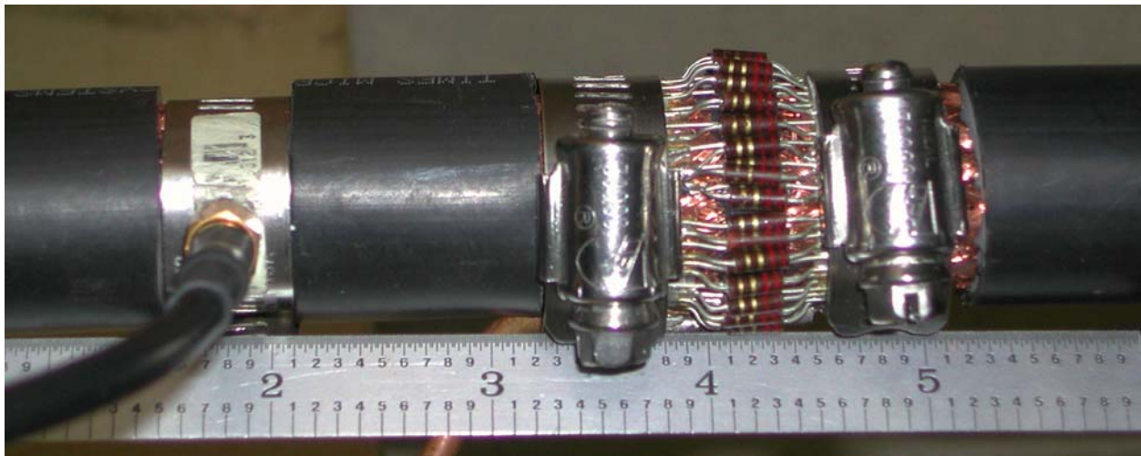
Figure 3.4. SMA sensor (left) and CVR sensor (right) installed onto the Marx output cable.
