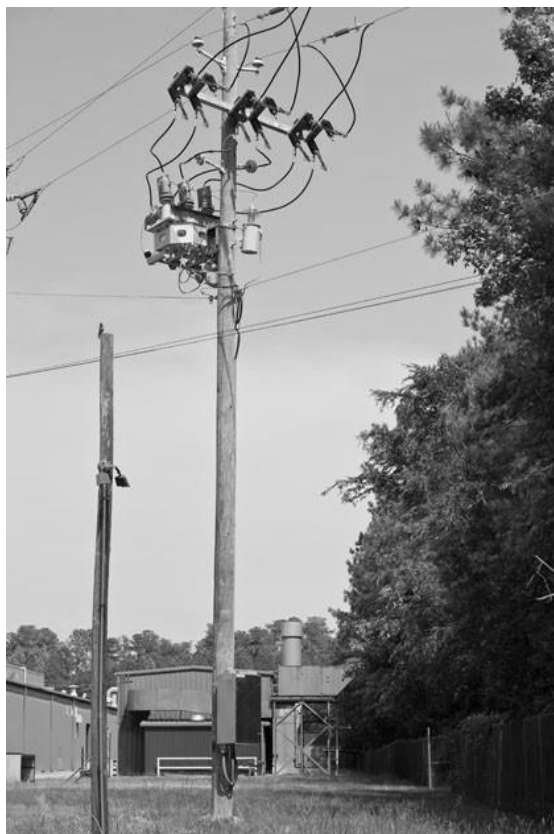
Figure 7. Reclosers on a Pole
