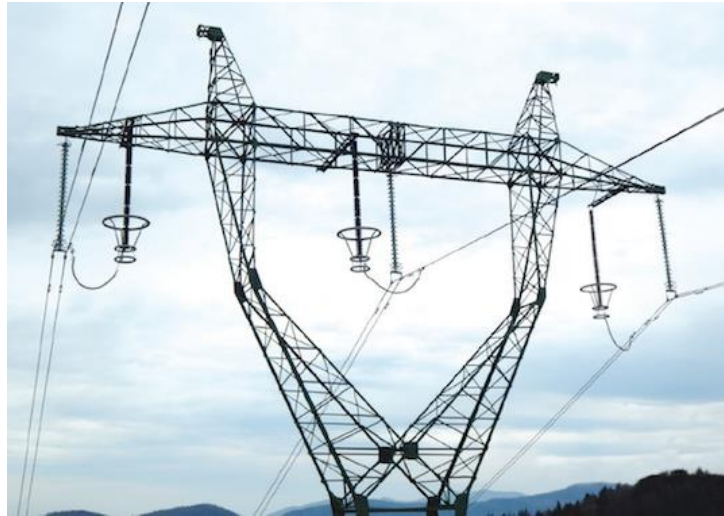
Figure 11. Romanian Tower-Mounted 400kV Transmission Line Arresters (with grading rings)
