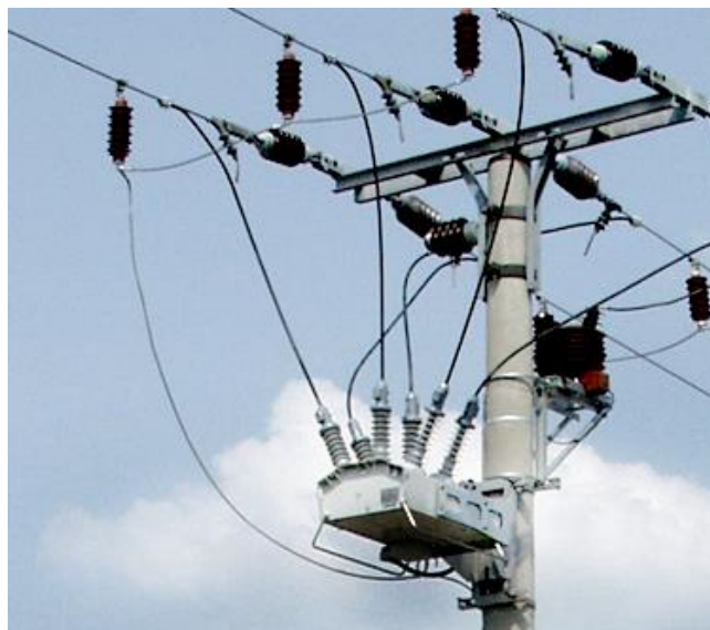
Figure 8. Pole Mounted Recloser
