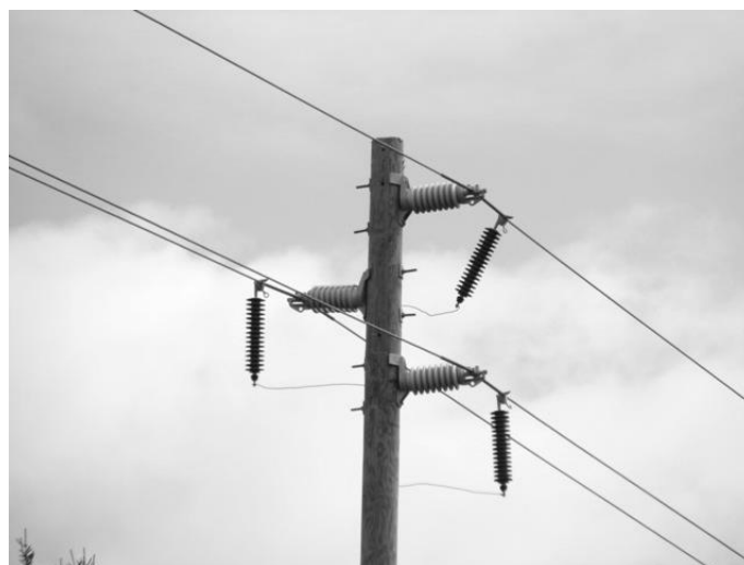
Figure 10. Transmission Line Arrestors
