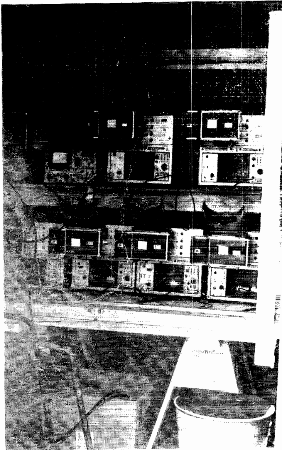
FIGURE 10 INTERIOR VIEW OF INSTRUMENTATION TRAILER
